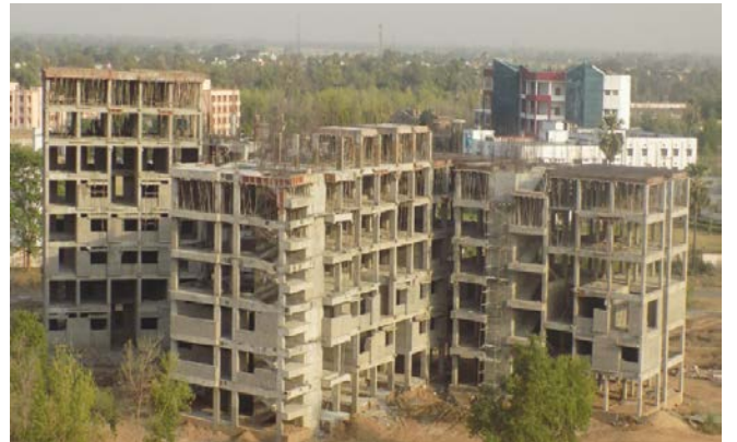
Boys Hostel (Capacity: 450 capacity) 45% complete (RCC of 6 th and 7 th floor is in progress)
